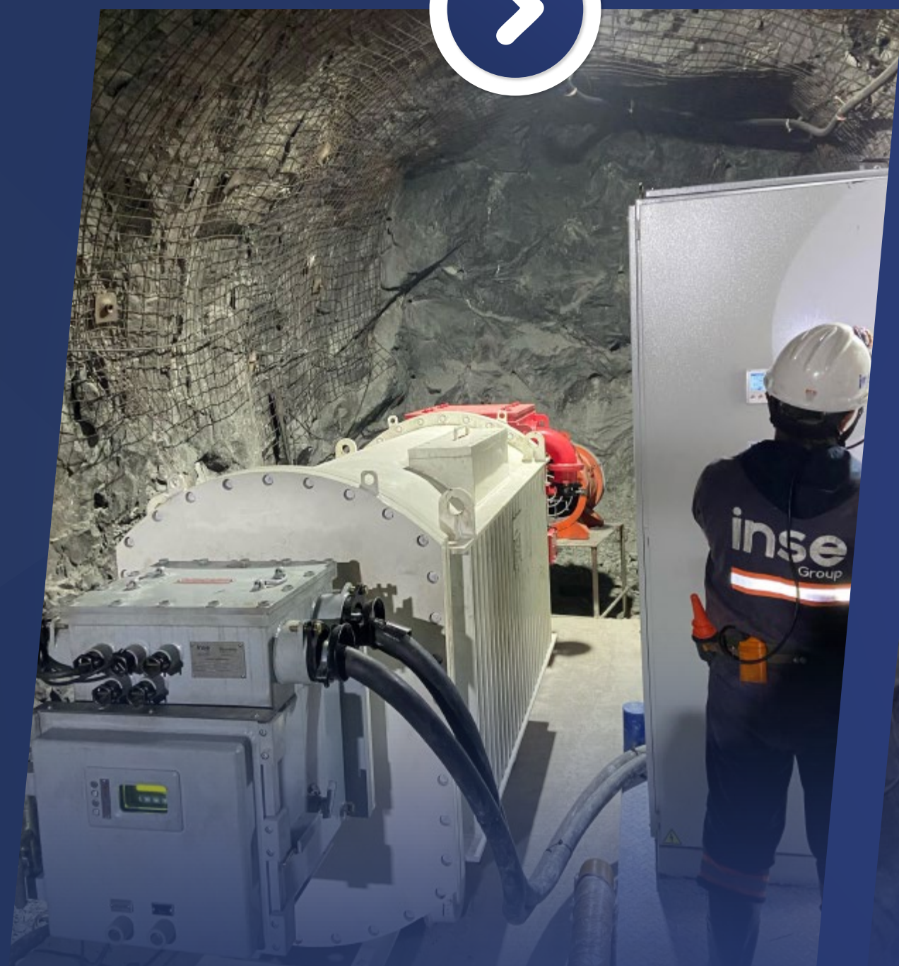
Annual preventive maintenance for electrical systems
